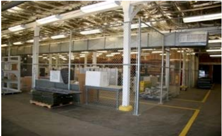
Fencing Installed to Secure Radio Equipment as a Result of Our Audit
